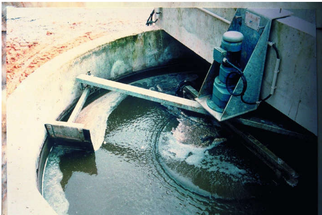
Figure 277. Circular grit/grease separator.
