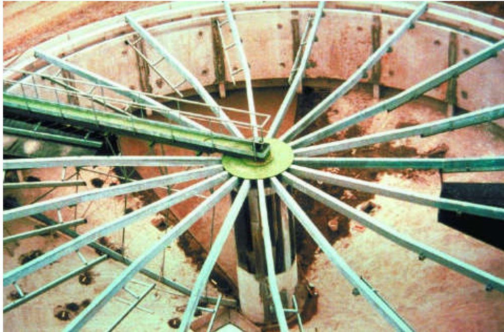
Figure 362. Maxéville (Eastern France) facility for the Champigneulles brewery. Flow rate: 600 \text{ m}^3 \text{ h}^{-1} . One of two 20 m dia. Rotation units.
