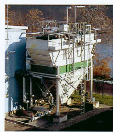
Figure 317. Metal Sédipac. Facility in Rheinfelden, Germany.
