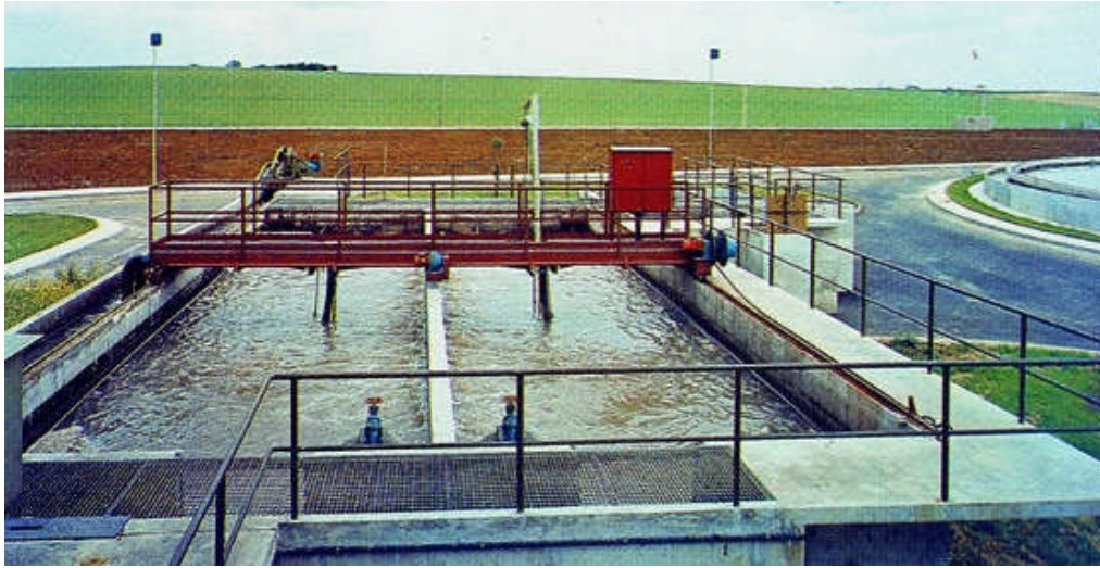
Figure 271. Aerated rectangular grit chamber.
