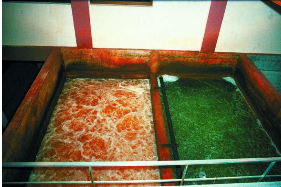
Figure 410. Métabief facility, France. Maximum flow: 2,300 \text{ m}^3 \cdot \text{d}^{-1} . MW purification. 4 Biofor reactors with 10.5 \text{ m}^2 unit surface area.
