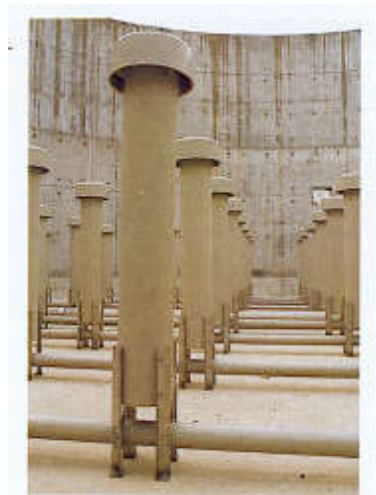
Figure 387. Tariscon facility in southern France for Cellulose du Rhône. Flow: 36,000 \text{ m}^3 \text{ d}^{-1} . Deep aeration tank with Dipairs.
