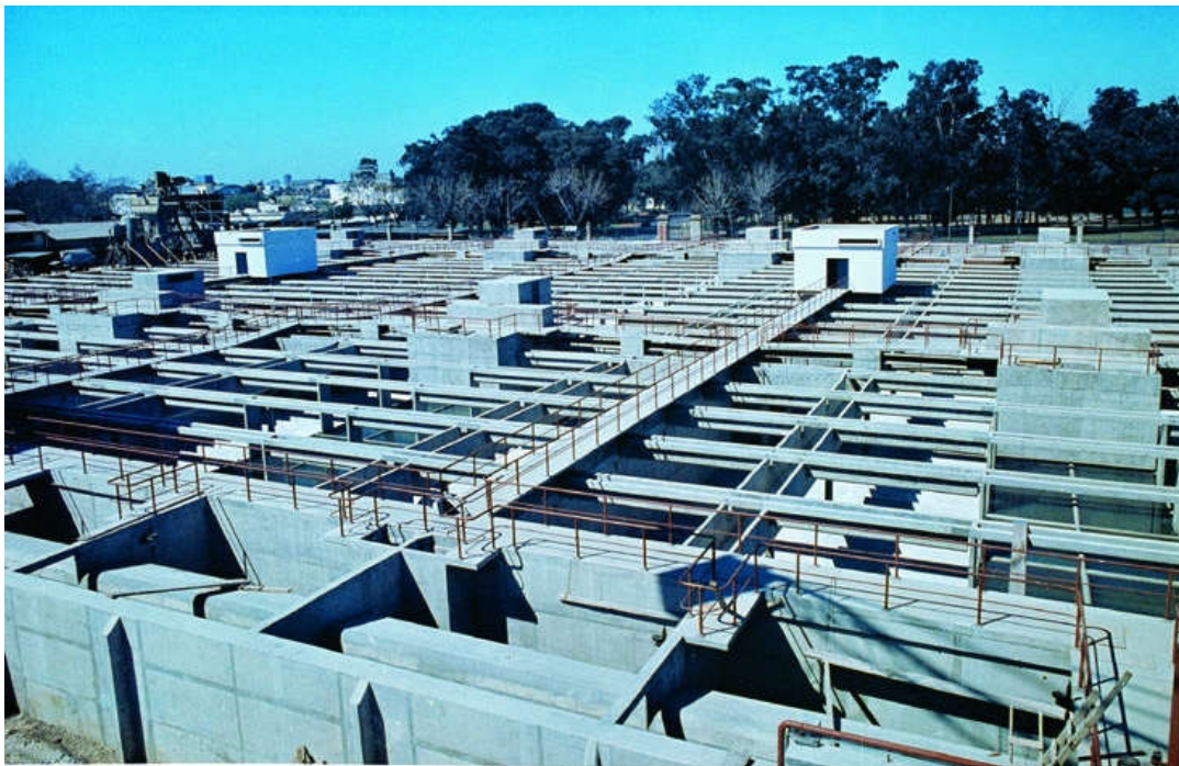
Figure 333. Palermo II facility for drinking water supply for Buenos Aires (Argentina). Flow: 36,000 m 3 .h -1 . Surface water clarification. Four Pulsator clarifiers, 99.5m x 27 m.
