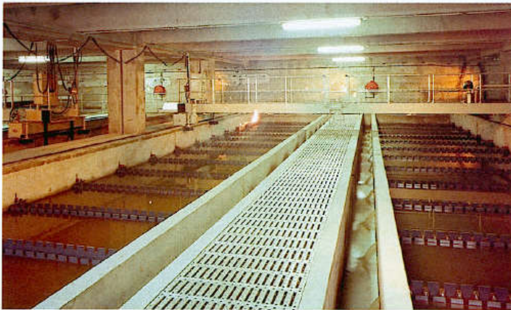
Figure 320. Facility in Nice (Southern France). Flow rate: 220,000 \text{ m}^3 \cdot \text{d}^{-1} . General view of a Sédipac U unit: 7 \times 21.1 \text{ m} .
