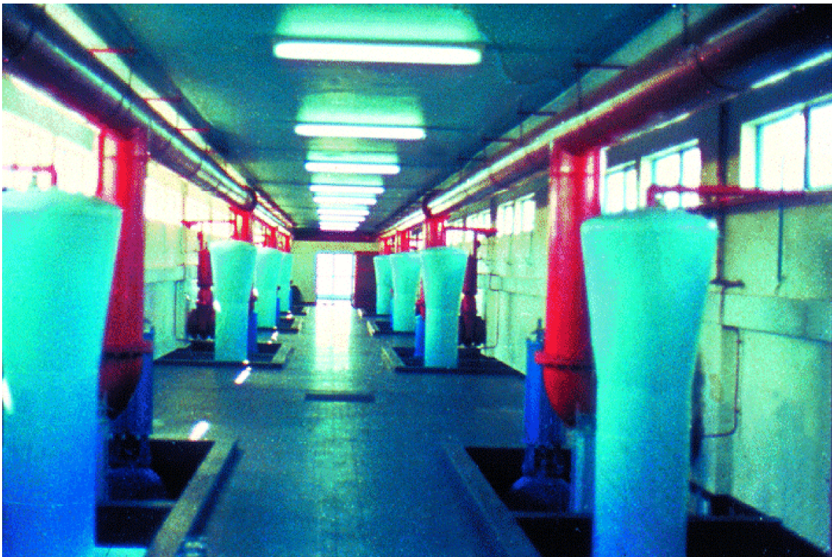
Figure 479. Brasilia facility, Brazil. Capacity: 5,000 \text{ m}^3 \cdot \text{h}^{-1} . Surface water clarification. Siphon gallery.
