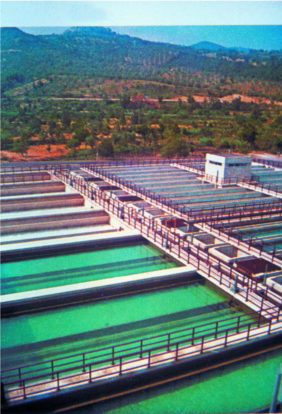
Figure 453. Treatment plant at Pertusillo (Italy). Battery of 14 double Aquazur V filters. Capacity: 16,200 \text{ m}^3 \cdot \text{h}^{-1} .
