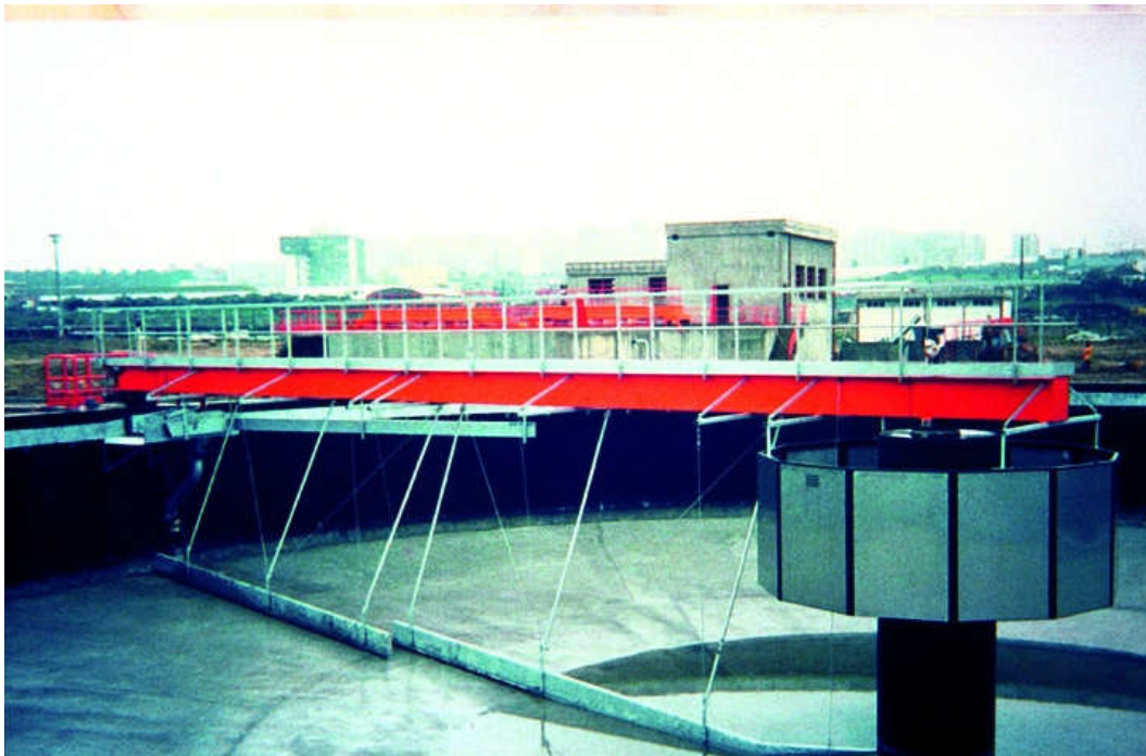
Figure 305. Type P circular scraper settling tank. General view.
