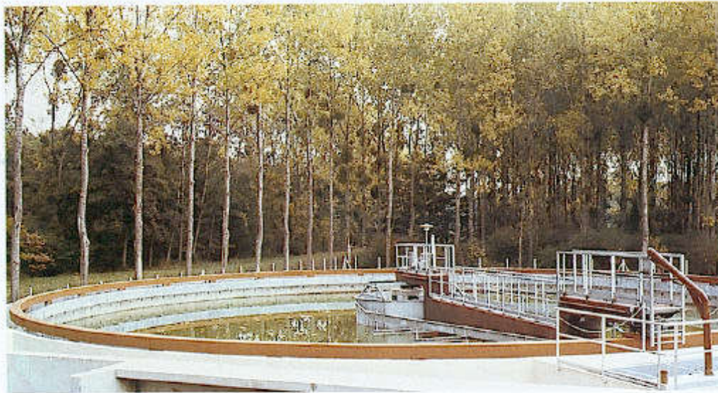
Figure 322. Zellwiller (Eastern France) facility. SV-type settling tank.
