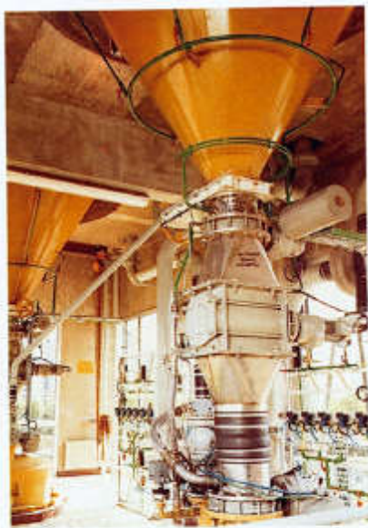
Figure 97. Facility in the city of Nantes (western France). Flow: 11,700 \text{ m}^3 \cdot \text{h}^{-1} . PAC feed unit.
