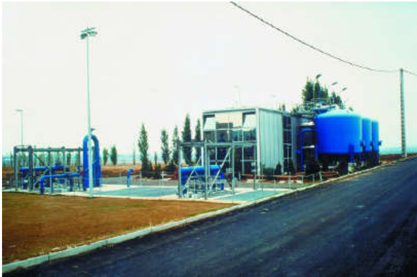
Figure 417. Obernai facility for the Kronenbourg brewery in eastern France. Flow: 15,000 m 3 .d -1 . Tertiary treatment by filtration ow Biolite with predissolution of air.
