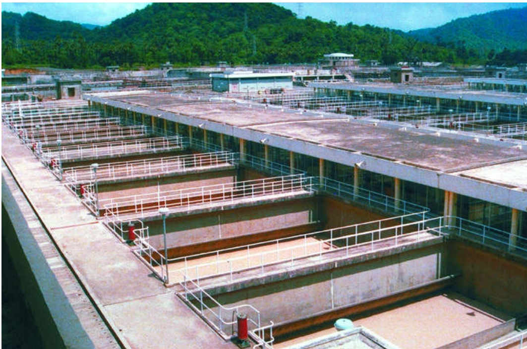
Figure 474. Bombay 1 plant (India), Maximum capacity: 87,500 \text{ m}^3 \text{ h}^{-1} . Production of drinking water. 72 declining rate Aquazur V filters. Surface area per unit: 151.4 \text{ m}^2 .
