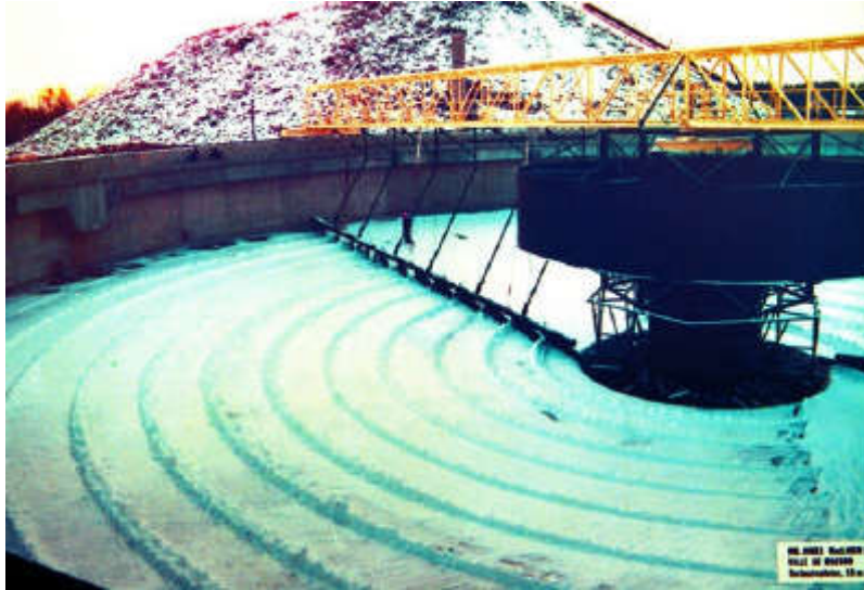
Figure 342. James MacLaren Industries Inc. (Canada). Primary settling of effluents. Turbocirculator 55 m dia.
