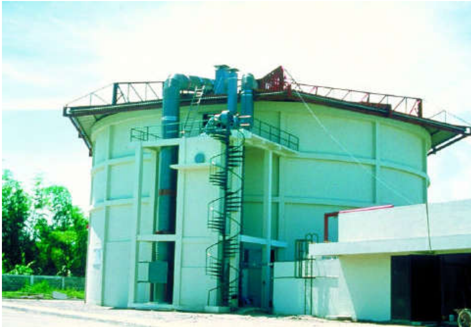
Figure 406. San Miguel brewery, Philippines. Capacity: 14 t BOD 5 per day. Trickling filter for pretreatment.
