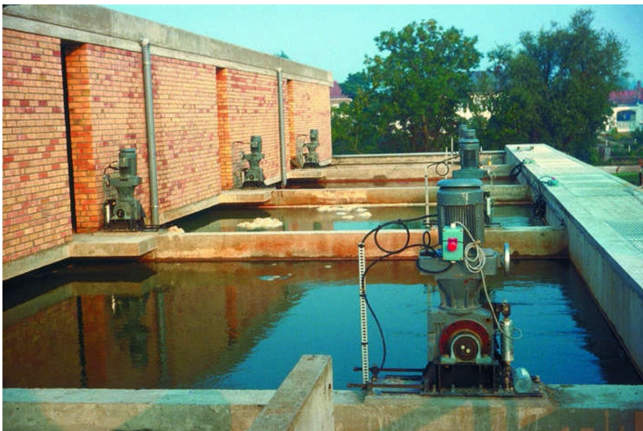
Figure 302. Moule facility (Northern France) for LE-Dumez. Surface water clarification by flotation. Battery of four dual-cell flocculators: Flow: 4 \times 300 \text{ m}^3 \cdot \text{h}^{-1} .
