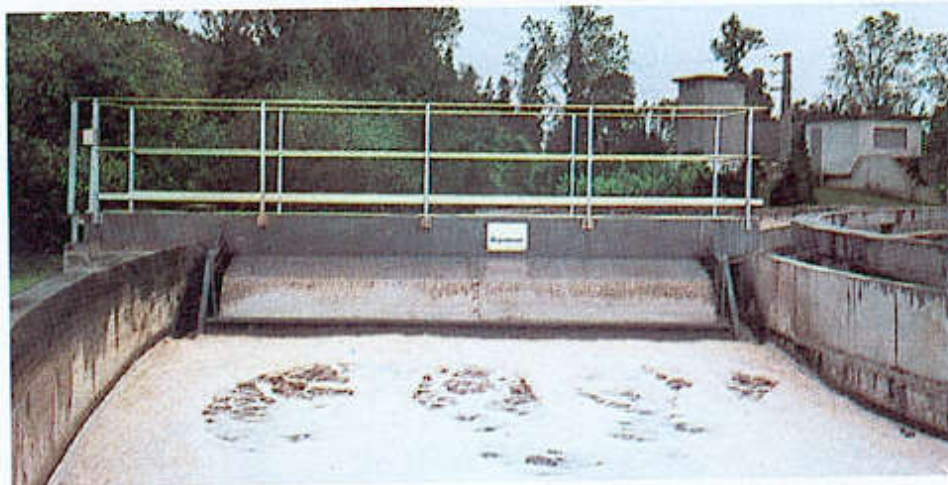
Figure 379. Rollox type 740 installed in an oxidation ditch.
