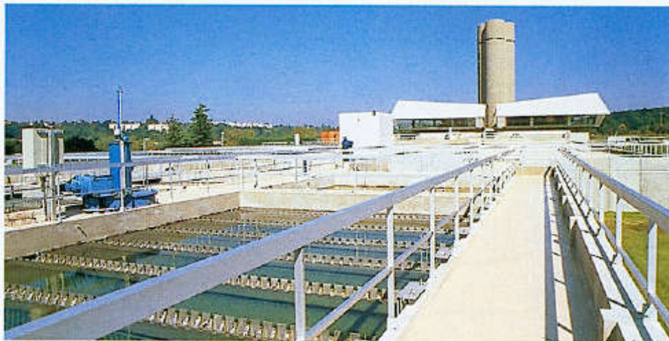
Figure 347. Extension of the LE-Dumez facility in Morsang-sur-Seine (Paris area, France). Clarification of water from the River Seine. Flow rate: 3,800 \text{ m}^3 \cdot \text{h}^{-1} . RL Densadeg clarifier. Settling velocity in the lamellae zone: 22.5 \text{ m}^3 \cdot \text{h}^{-1} .
