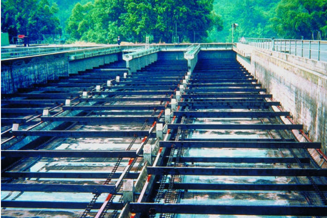
Figure 313. Aire effluent treatment facility in Geneva (Switzerland). Flow rate: 3.6 \text{ m}^3 \cdot \text{s}^{-1} . One of the 8 settling tanks equipped with a flight-and-chain scraper system. Dimensions: 70 m x 18.5 m.
