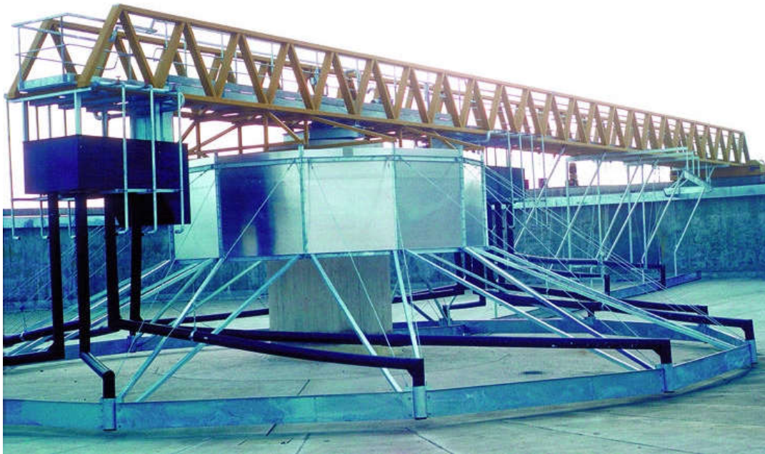
Figure 326 Roanne (Central France) facility. Flow: 30,000 \text{ m}^3 \cdot \text{d}^{-1} Succir type settling tank, 54 m dia.
