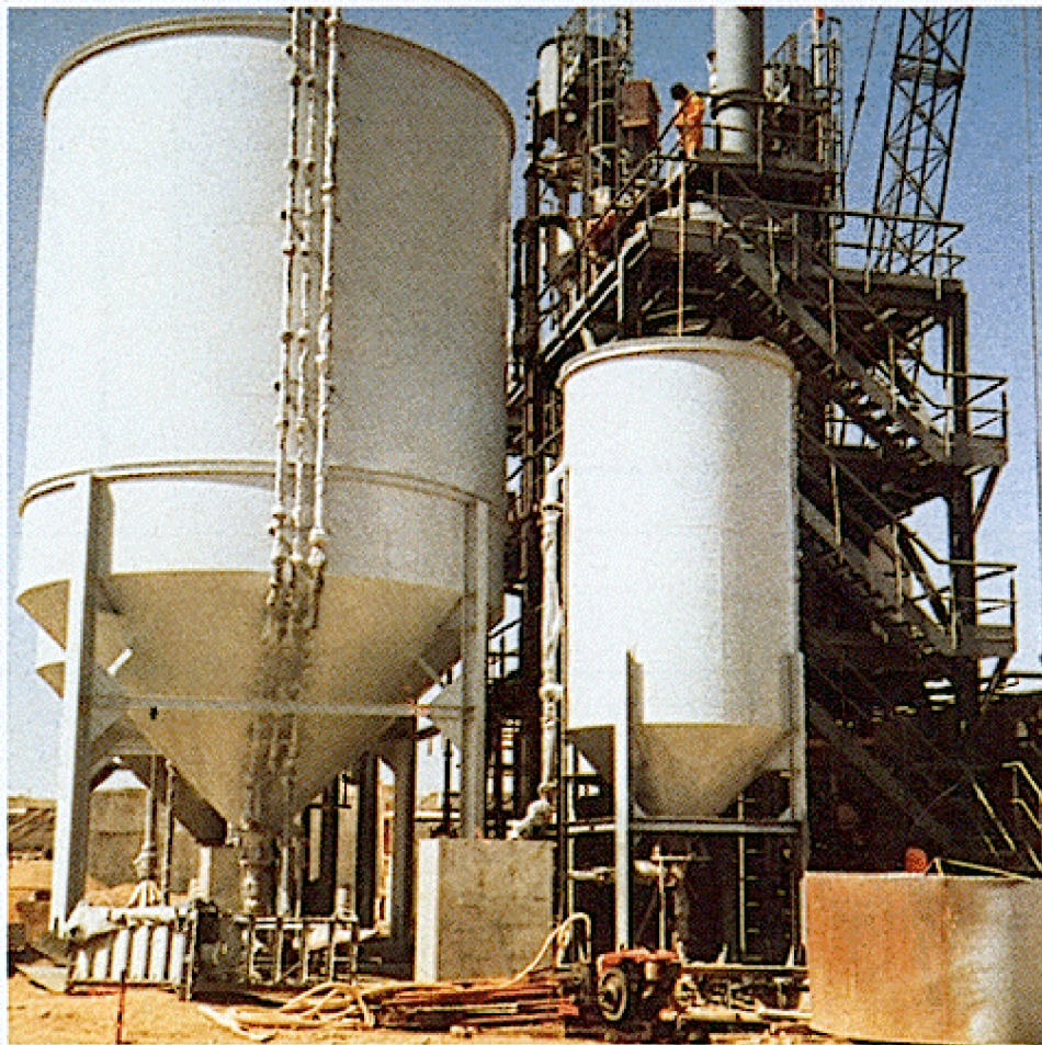
Figure 101. Taif facility (Saudi Arabia). Flow: 12,600 \text{ m}^3 \cdot \text{d}^{-1} . GAC regeneration furnace. Capacity: 6 \text{ t} \cdot \text{d}^{-1} .
