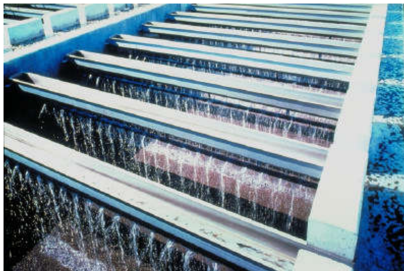
Figure 414. Mannheim facility, Germany. Polishing treatment for purification of municipal wastewater. Maximum flow: 14,000 \text{ m}^3 \cdot \text{h}^{-1} . 32 Biodrof reactors (unit surface area: 87 \text{ m}^2 ).
