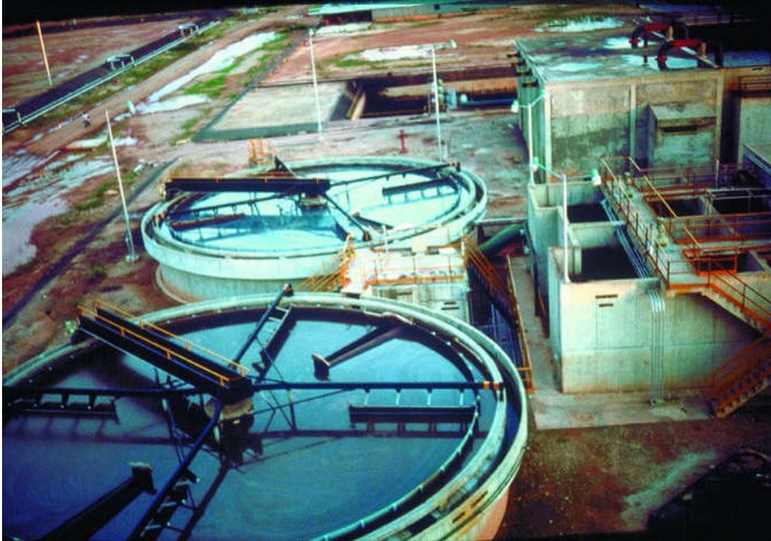
Figure 358. Barrancabermeja (Colombia) facility for Ecopetrol. Flow rate: 3,000 \text{ m}^3 \cdot \text{h}^{-1} . Flotation of oily water. 4 Sediflotazur units, each 15 m dia.
