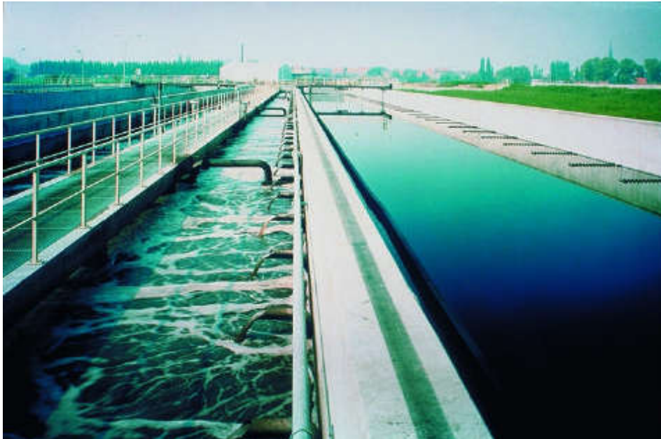
Figure 401. Harelbeke facility, Belgium. Purification of municipal wastewater by Oxyrapid R.
