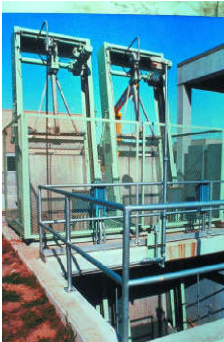
Figure 270. Vertical grab bar screens.
