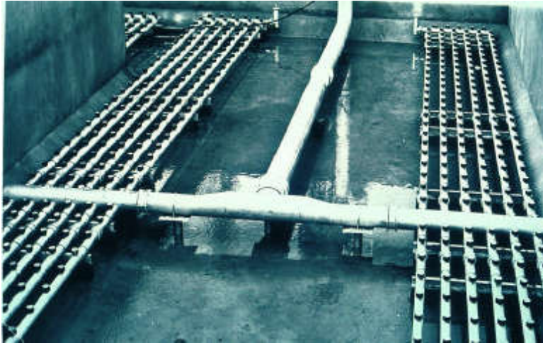
Figure 385. Aeration tank equipped with Vibrair diffusers.
