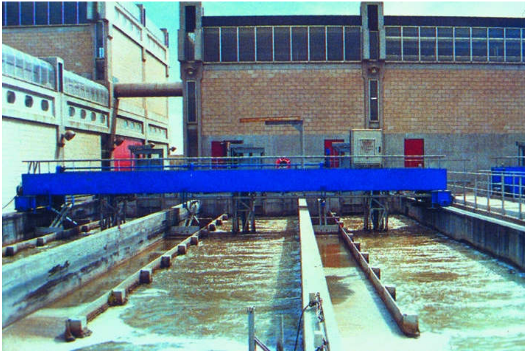
Figure 278. Rectangular grit/grease separators.
