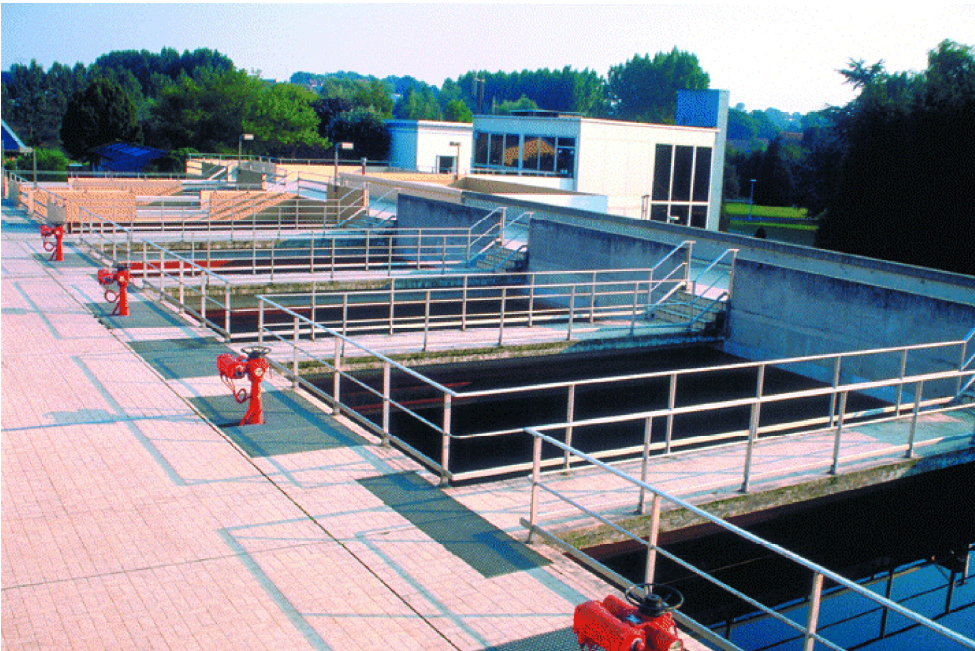
Figure 458. LE-Dumez facility at Moule (Northern France). Capacity: 2,000 \text{ m}^3 \cdot \text{h}^{-1} . Battery of seven Mediazur V filters for granular activated carbon filtration.
