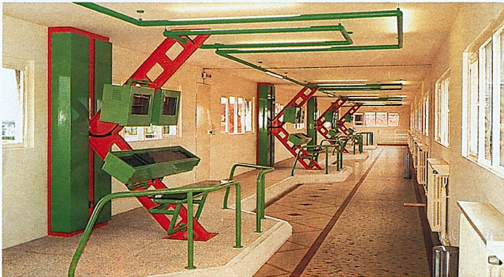
Figure 477. Mont Valérien facility (Paris area, France), for CEB. Clarification of Seine river water. Capacity: 2000 \text{ m}^3 \cdot \text{h}^{-1} . Filter control gallery for 12 Aquazur filters.
