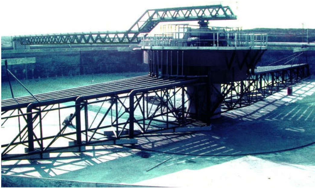
Figure 327. Valenton (Paris area, France) facility for SIAAP. Flow: 300,000 \text{ m}^3 \cdot \text{d}^{-1} . SD-type settling tank, 52 m dia.
