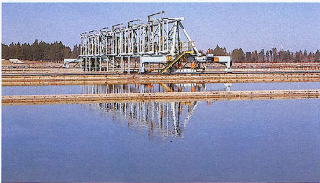
Figure 314. Settling tanks with scraper gantry serving multiple units (4 tanks, each 50 m x 200 m).
