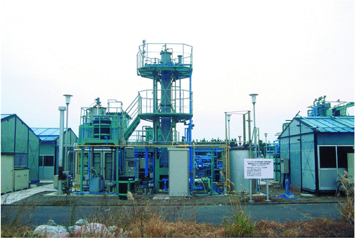
Figure 154. Methane fermentation pilot. Anaflux reactor.
