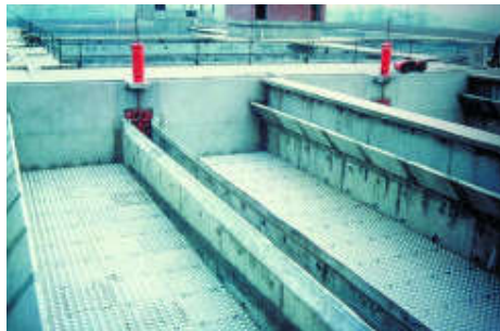
Figure 445. Aquazur V filters under construction: view of the filter floor with the nozzles, the V-shaped sweeping trough, and the wash water discharge trough.
