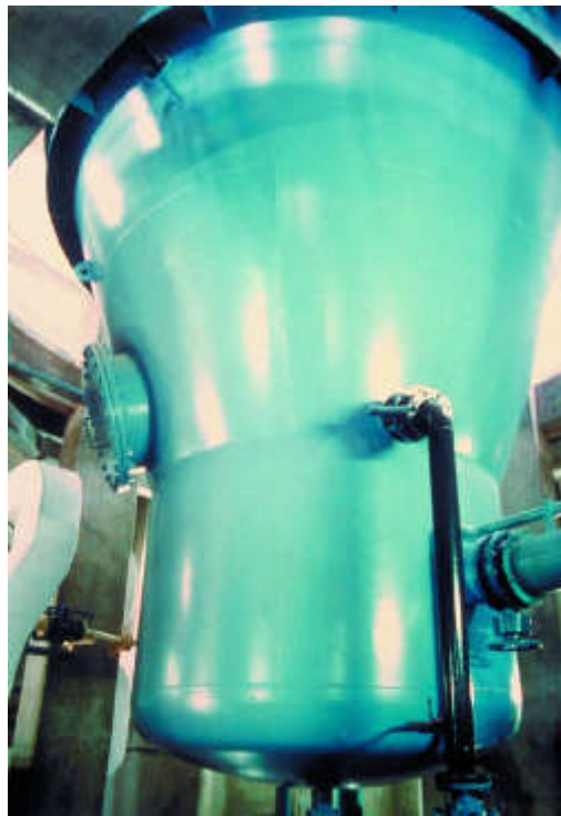
Figure 351. LE-Dumez facility in Villeneuve-la-Garenne (Paris area, France). Maximum flow rate: 1,800 m 3 .h -1 . Lime softening of groundwater using a Gyrazur reactor. View of the reagent feed point at the base of the unit.
