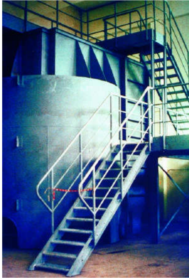
Figure 348. Franken 11 (Germany) facility. Flowrate: 150 \text{ m}^3 \cdot \text{h}^{-1} . Clarification of river water for the production of process water. Steel Densadeg clarifier.
