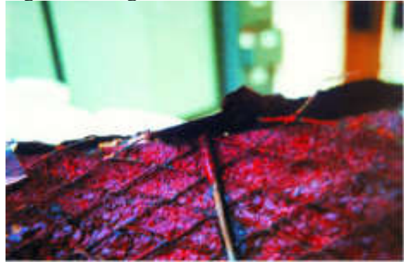
Figure 216. Example of serious external corrosion of concrete piping.
