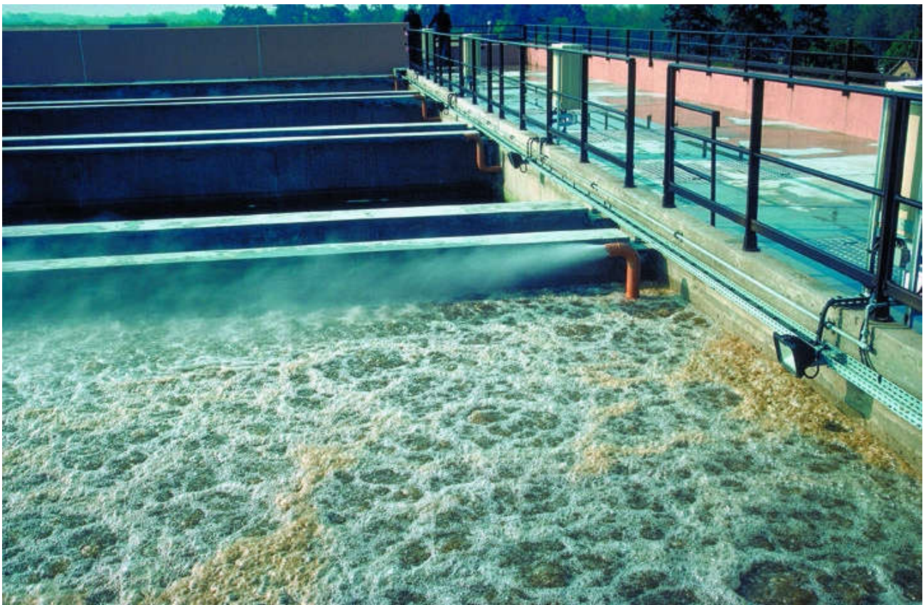
Figure 149. Fixed bed reactor (Nitrazur) being washed. Louveciennes plant near Paris (France). Nitrification of groundwater, Maximum flow: 5000 \text{ m}^3 \cdot \text{h}^{-1} .
