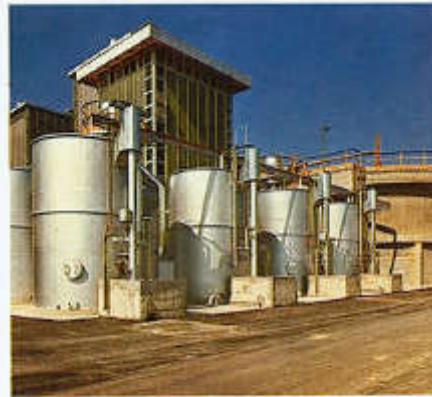
Figure 460. Facility at La Casella (Italy) for the Enel-La Casella thermal power plant. Capacity: 300 m 3 .h -1 .
